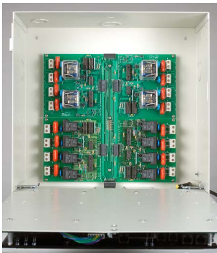
Flip the logic board down to access the line-voltage area on the Greengate lighting control panel (shown here)
